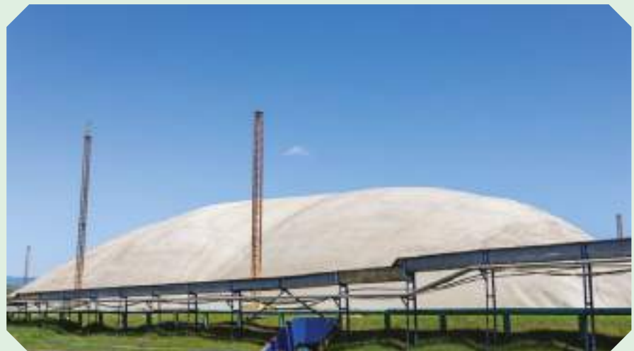
Anaerobic lagoons that capture biogas to transform it into electrical energy
